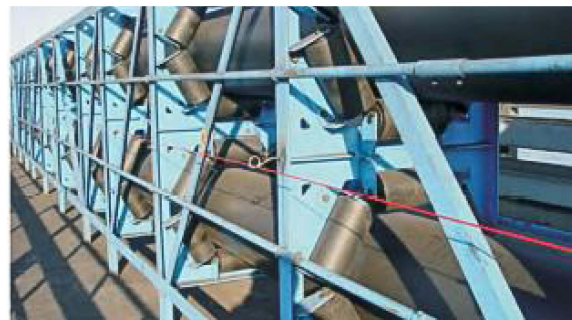
Pipe Belt Conveyor
