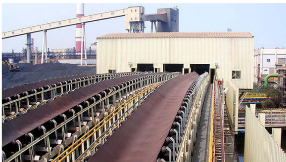
General Belt Conveyor
